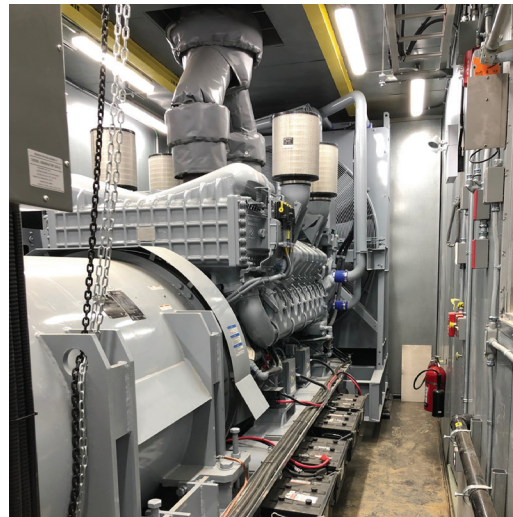
One of three Power Plant Gen Sets.
