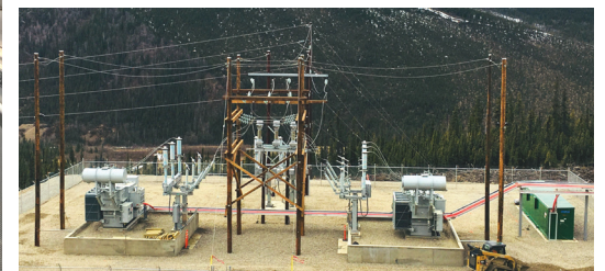
Mine site sub-station.
