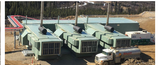
Diesel power plant being commissioned.
