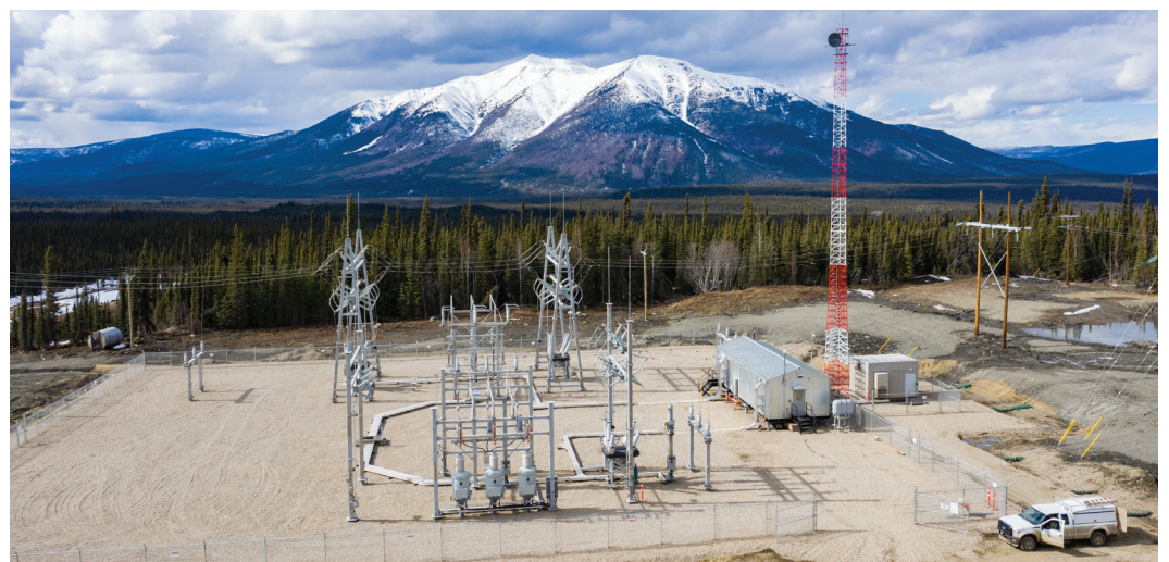
McQuesten Sub Station.
